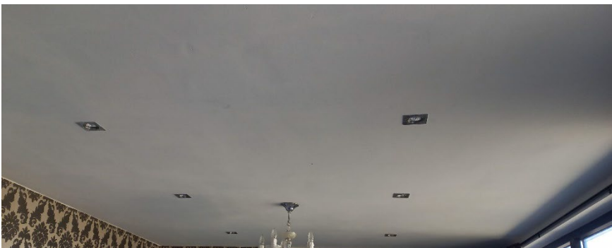
Figure 3. Picture of a roof of one of the camping cabins with halogen lamps.
